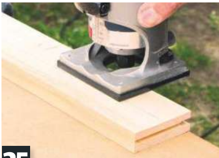
25 Door panels are from 6mm MDF. Rout groove around inner edges of rails and stiles with slotting cutter
